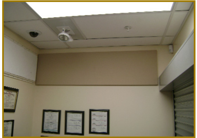
Above: This picture shows how the installer was able to site fabricate a wall panel to specific dimensions. The ability to build panels specific to the size of the available wall space is a great way to fit acoustical panels into an existing room where the installation looks intentional.
